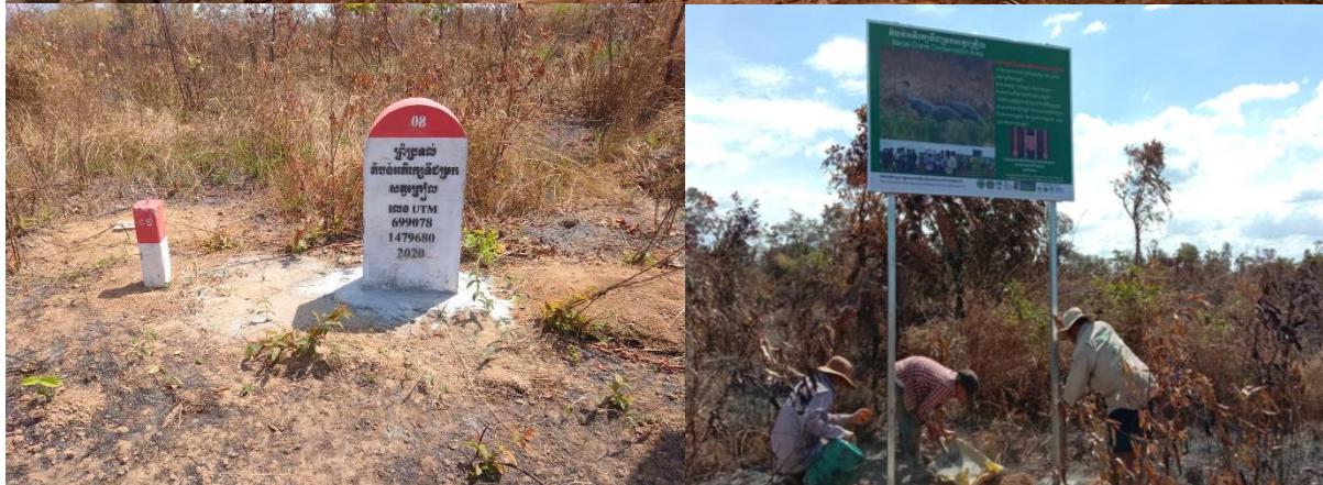
Boundary pole installation around a land plot that agreed to keep for critically bird habitat in Hoang Anh Lumphat.
