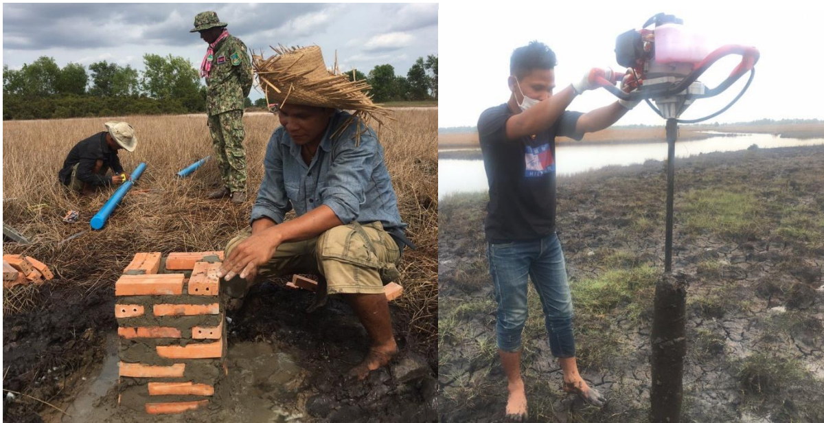
Floodwater gauges were installed in AP and 4 in BPL to measure the level of water during the wet season.
